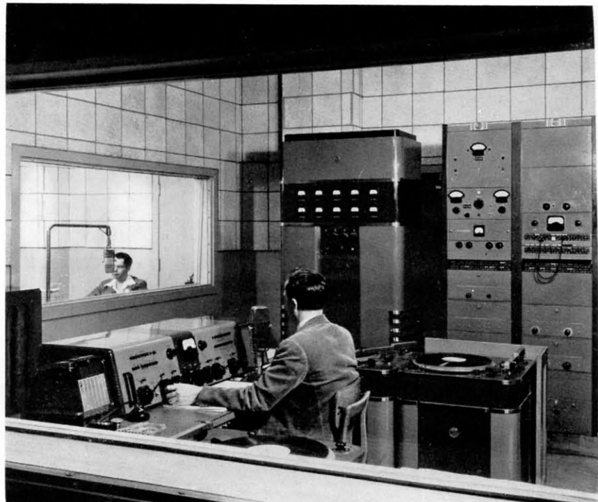
FIG. 6. The main control room houses the transmitter and studio equipment which is one hundred percent RCA.
