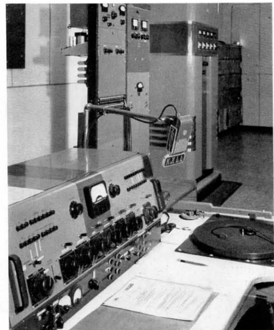
FIG. 3. The control console and transmitter are so placed that the operator can easily monitor all the equipment.
