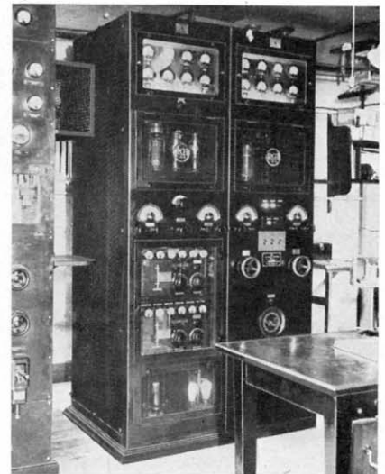
THE NEW RCA 1-C TRANSMITTER AT WBEN.
