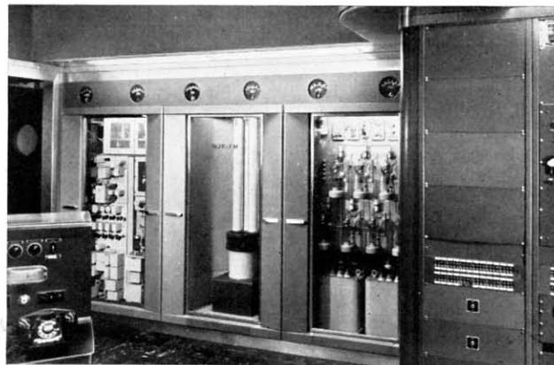
New FM transmitter at WJR is installed in master control room for ease of operation.
