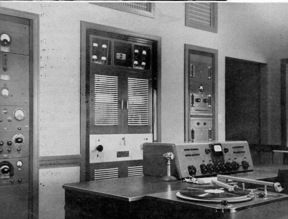
▲ A DeLuxe 250 D installation at WSPB, Sarasota, Fla. One of the South's finest "RCA-All-The-Way" installations.
