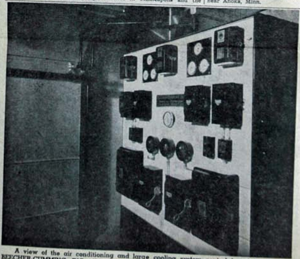
A view of the air conditioning and large cooling system control board installed by BEECHER-CUMMING, INC., distributors of Westinghouse products and appliances.
