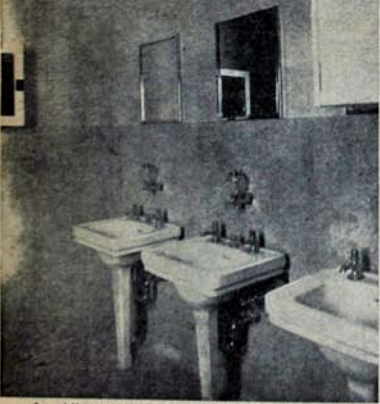
In addition to lavatories and wash rooms on each floor there are also shower rooms. The plumbing and heating work was installed by GRUDEM BROS. CO.
