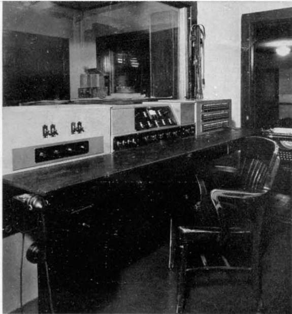
Portion of transmitter room showing studio speech input equipment.
