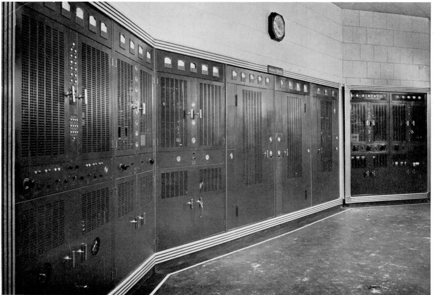
Line-up of WHN's transmitter panels showing (left to right) the 5 KW driver, 50 KW final amplifier and 1 KW auxiliary transmitter
