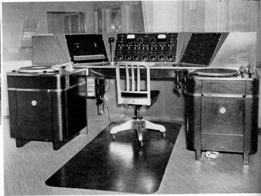
Seated at this control turret the operator has a clear view of both studios and of three racks of speech input equipment.
