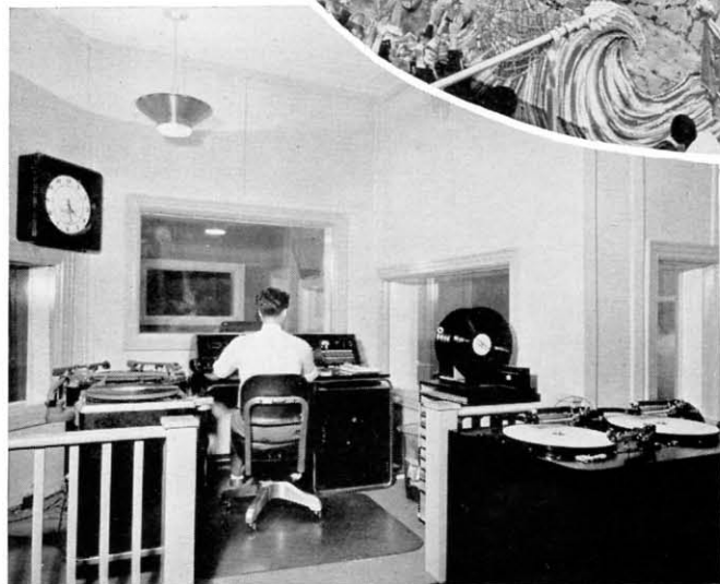
Above: Control Room for Studios A & B. Equipped with 80-AX Desk.
