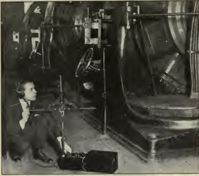
LARGE MOTORS AND GENERATORS
