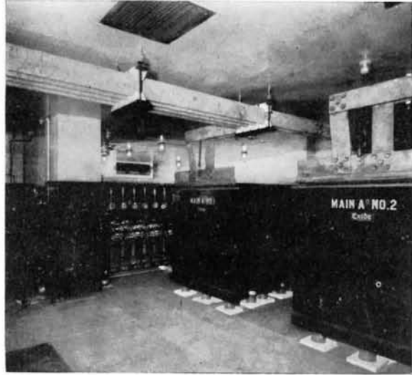
Figure 33. Fifty tons of storage batteries, "A" and "B," which are operated float-charge with the motor-generator sets in the power room.
