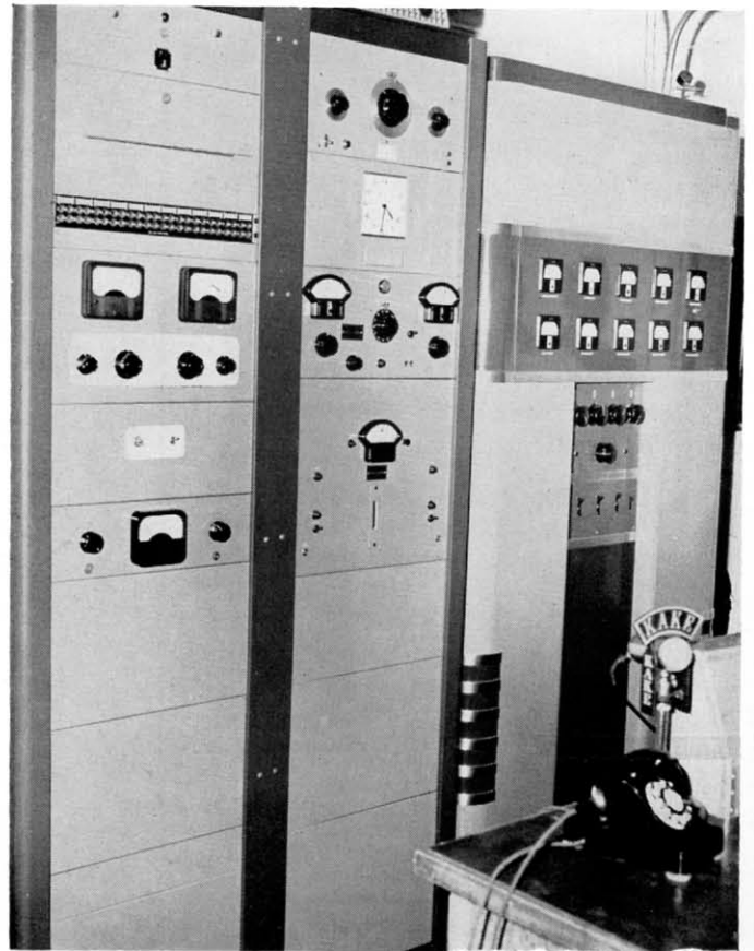
FIG. 1. KAKE's 250 W transmitter, RCA Type BTA-250L, is installed next to monitoring, test and audio equipment racks for convenient grouping.
