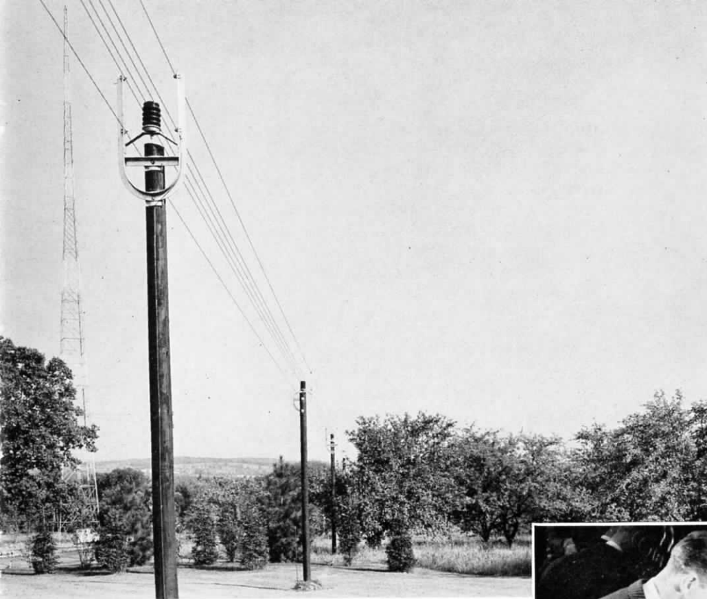
ABOVE: Six wire transmission line installed at WSYR, Syracuse. A complete description of this equipment appeared in the May issue of Broadcast News.
