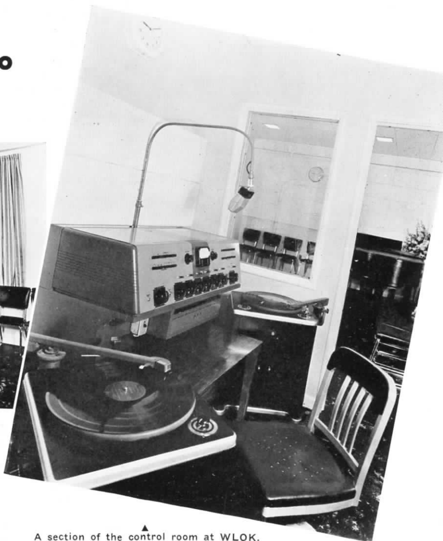
▲ A section of the control room at WLOK.
