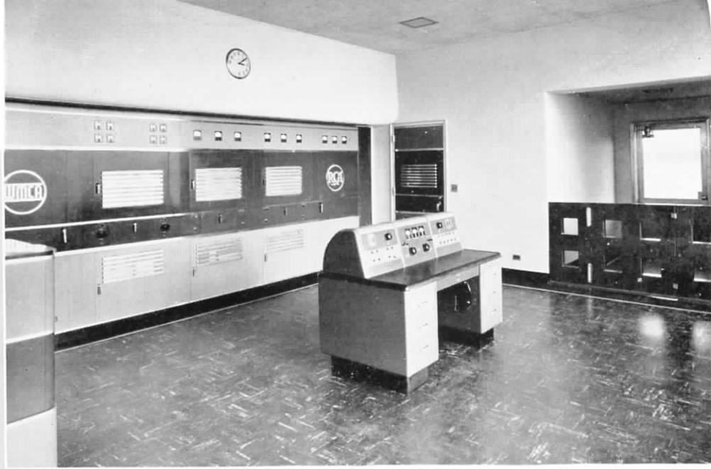
▲ The streamlined RCA 5-DX, 5 KW Transmitter, installed at WMCA with its associated control desk.
